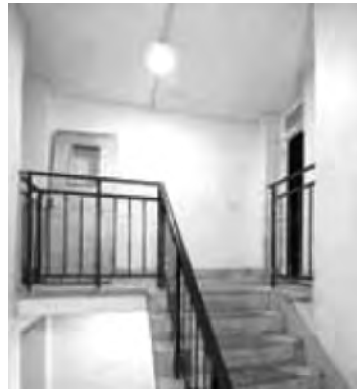
photo of stairwell with LED fitting
